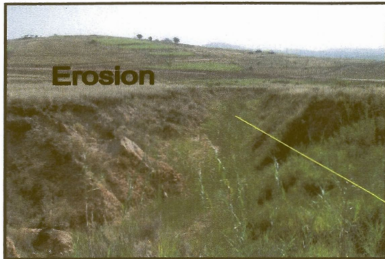
Figure 91: Erosion downstream at the Uvova site.
