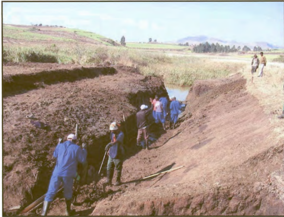
Figure 25: Before flooding. Photo taken downstream on 4 July 2002 at the Amatigulu site.
