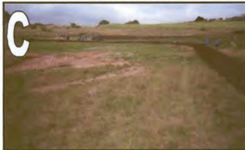
C Earthen embankment (500 mm) high storm drain to keep floodwater away from headcut on left. Large earthen embankment and buttress weir visible on top left of photo.
