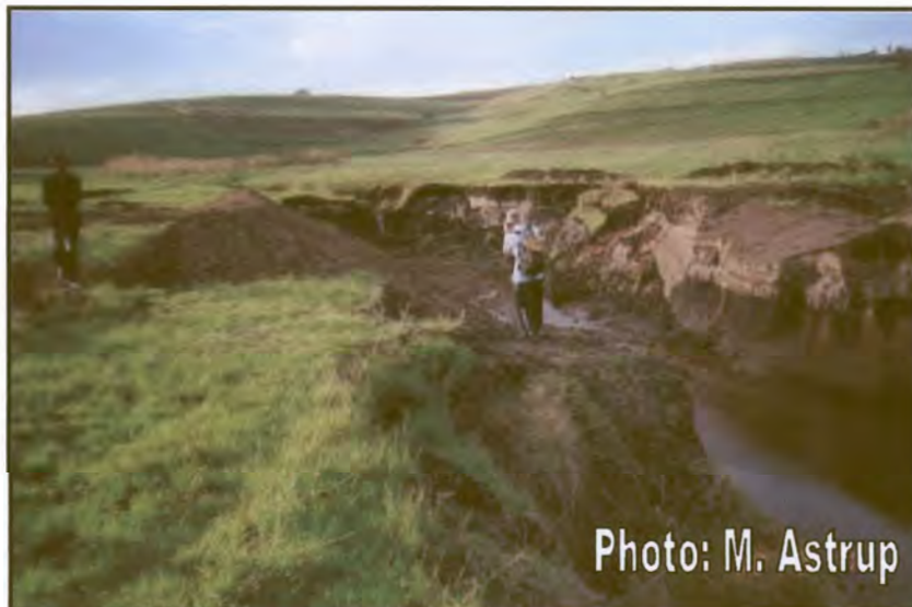
Figure 24: Amatigulu site. View of the damaged geocell chute after July 2002 floods. Note the lush green grass after the rains.
