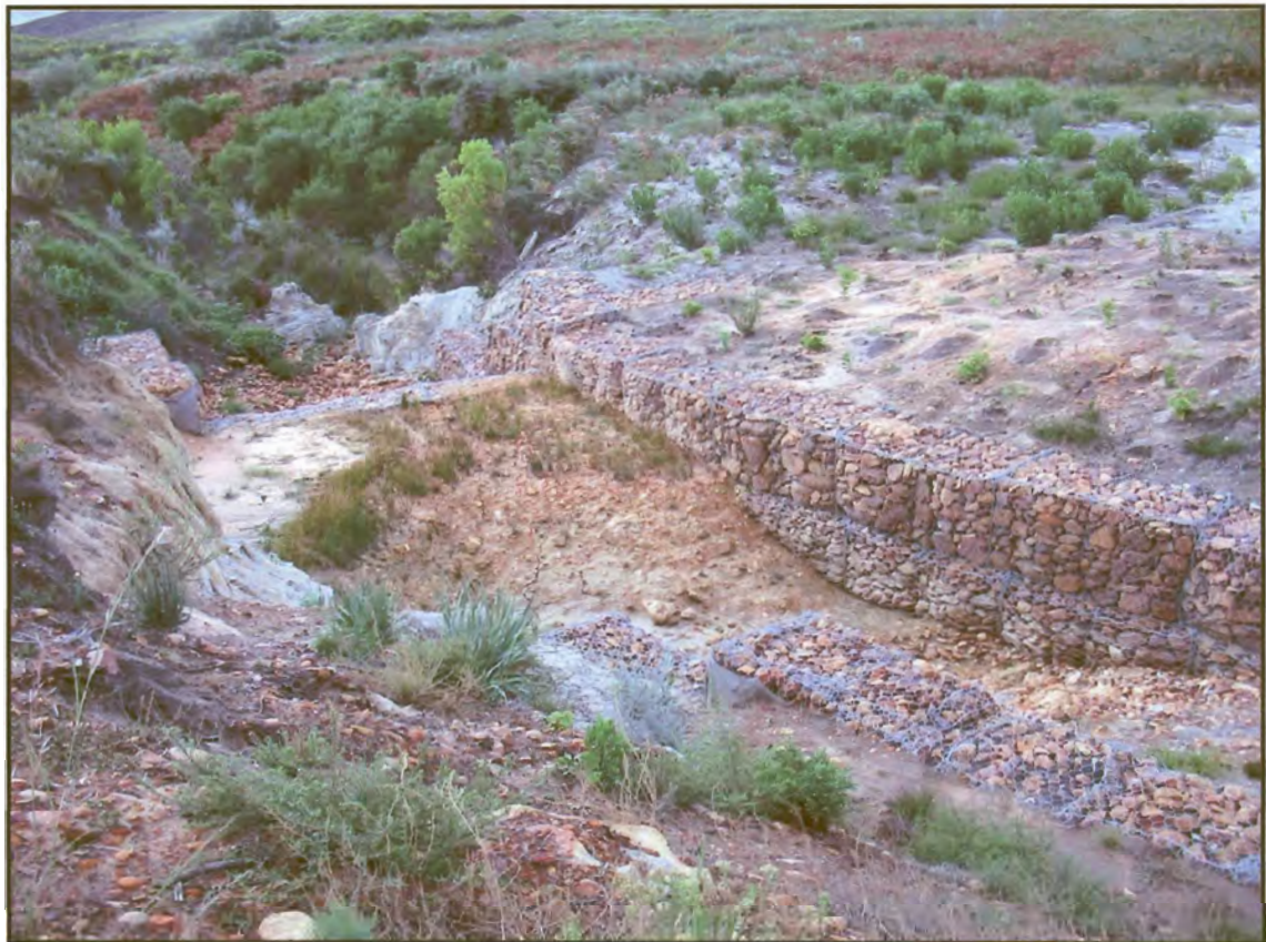
Figure 11: Close-up photo of the headcut rehabilitation structure at a tributary of the Kromme River. This rehabilitation structure will not form part of the Wilge River Wetland study but indicates rehabilitation measures in the catchment.
