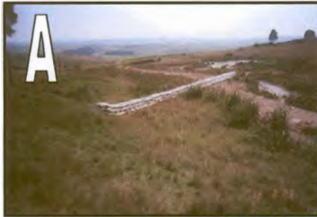
A Sandbag groyne to divert stream to right-hand course away from headcut. This is a temporary structure while stream formalizes channel to the right.
