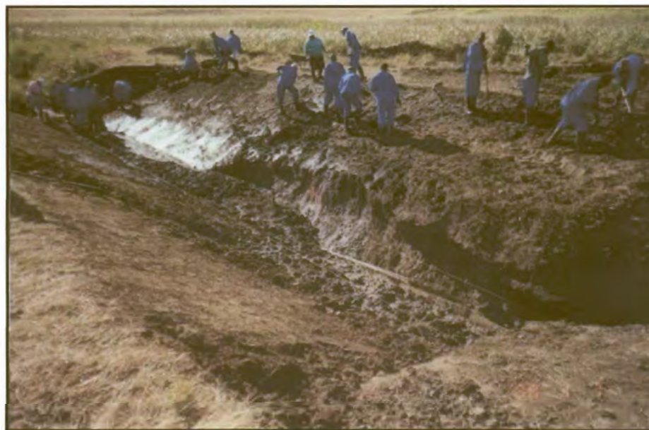
Figure 28: After flooding. Photo taken upstream after July 2002 at the Amatigulu site. Geocell chute preparation at 1:5 gradient (Photo: M. Astrup).
