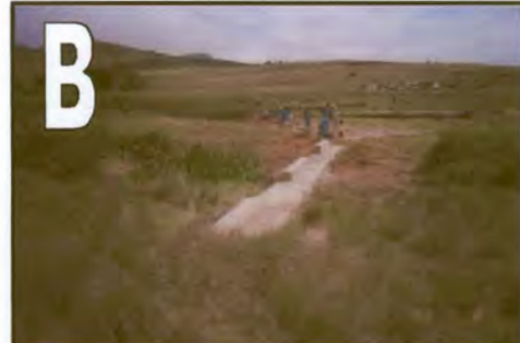
B Buttress weir under construction. 50mm PVC piping will carry base flow into headcut site.
