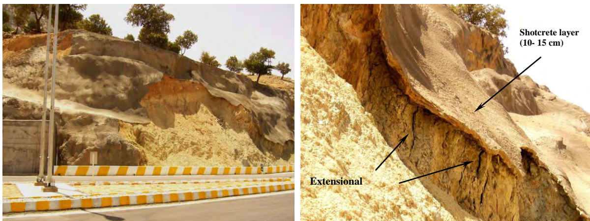
Figure 6.13. Rock slope failure after application of unreinforced shotcrete on marl units of the Asmari Formation. The marls or such rocks need to be stabilized by reinforced shotcrete due to ductility and deformability of the rock mass. The vertical extensional joints and fractures due to gravity movement of the rock mass can clearly be observed (Karun-3 dam site, entrance gate, 2007).
