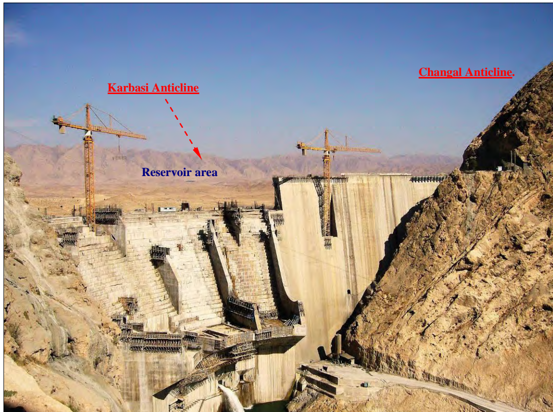
Figure 4.6.2. Salman Farsi (Ghir) dam is a concrete arch gravity dam 125 m high and is under construction on the Ghareh Agahaj River.
