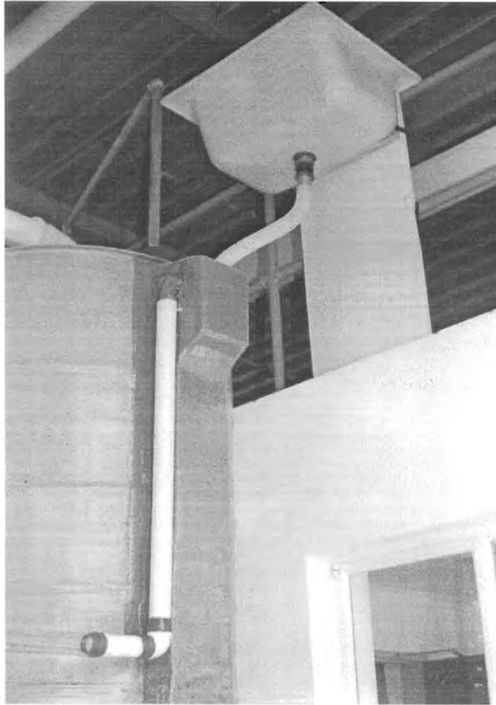
Figure 6.6: Working arrangement with washtub draining into the tank and siphonic outlet discharging into the pipeline (available hydraulic head between summit of siphon and outfall pipeline = 1,0m)
