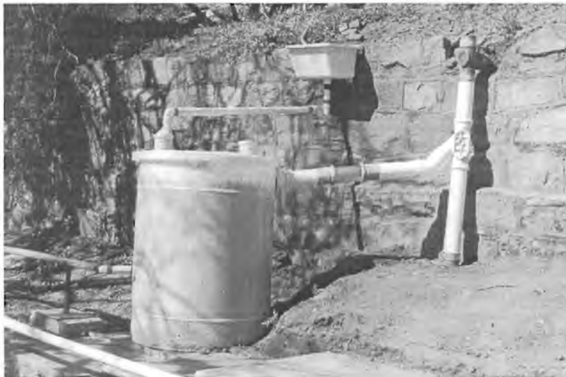
(b) Tank / washtub inlet and outlet assembly (before installation of valve in Y-junction)
