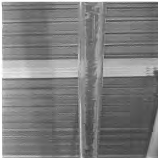
Figure 6.14: Actual septic tank sludge deposited on invert of pipeline after completion of flush (seen from underneath). Pipe gradient = 0,25 %; pipe ID = 46 mm.
