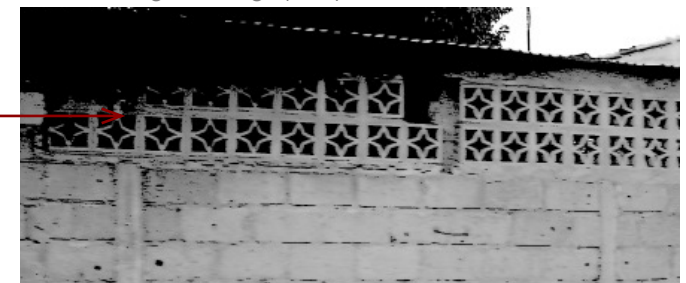
Figure 8.5 Photograph showing Concrete air clocks as ventilation and decoration. Photograph by Author 2011
