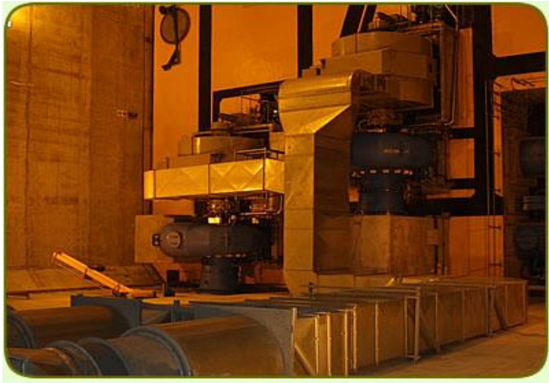
Figure 6: A Hydro Turbine at Dwaleni Power Station (Source: SEC; 2012)
